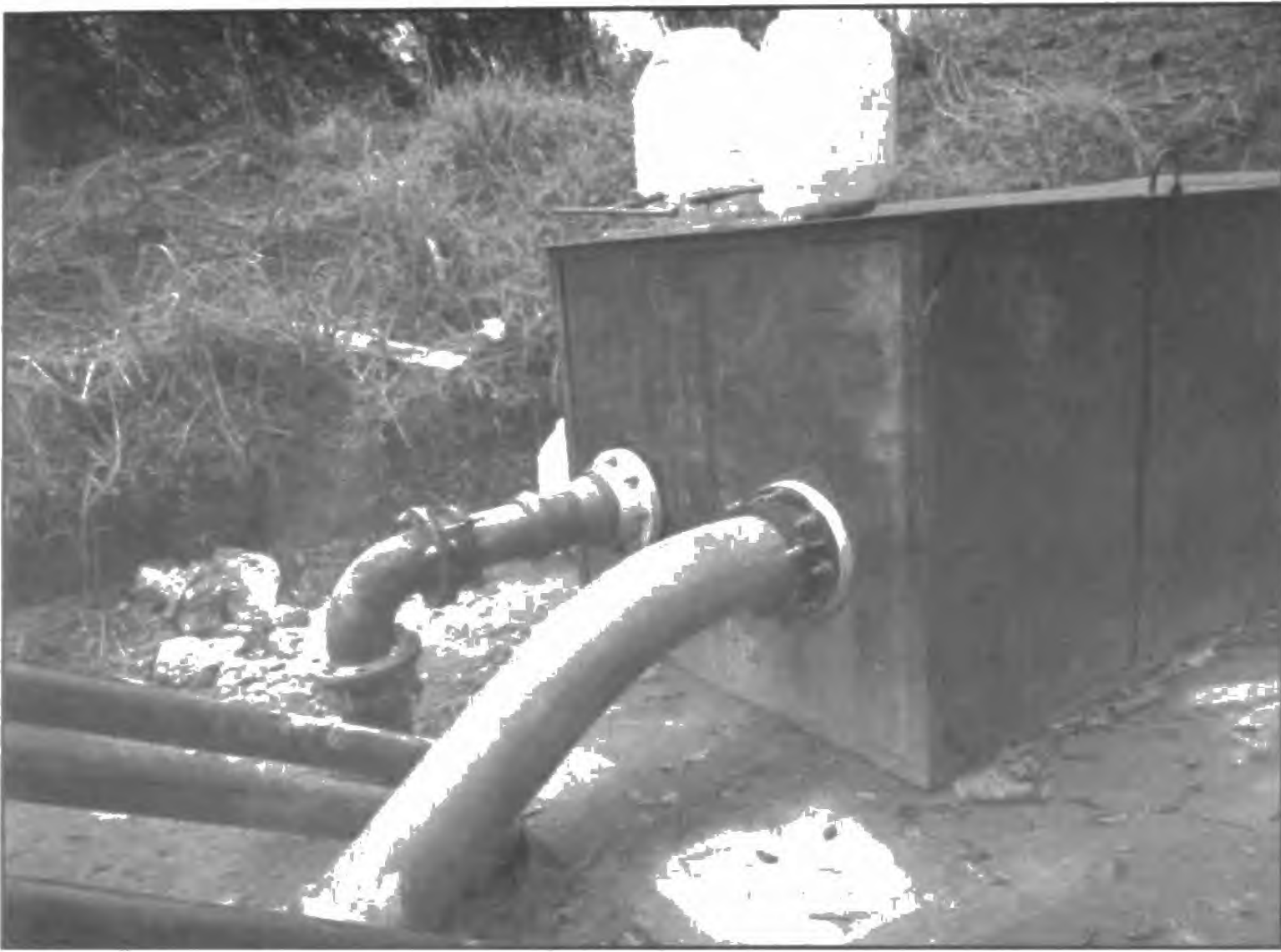
Figure 2: Installed Flocculator Unit
