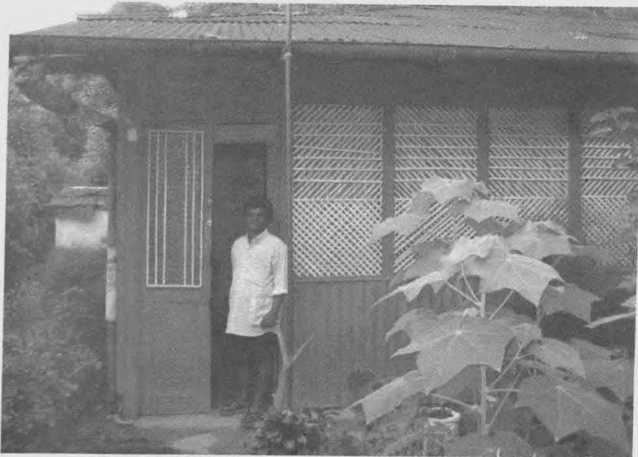
Figure 11: Affected Houses at Kumaragama Place, Talawakelle
