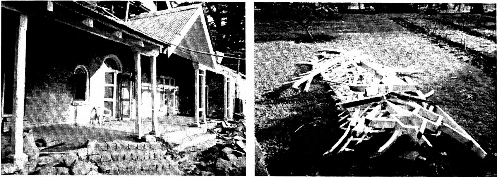
Fig. 15 & 16: Frontier House Back Side View and damaged wooden handrail Source: Author
