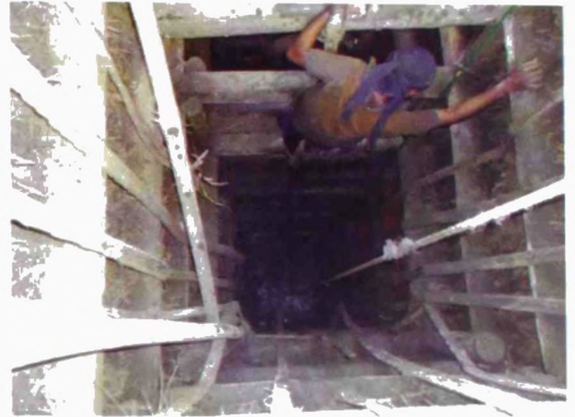
Plate 2 A part of a deep gem mine showing reinforcement with timber, mainly rubber wood. This reinforcement is done at about 3-4 ft intervals
