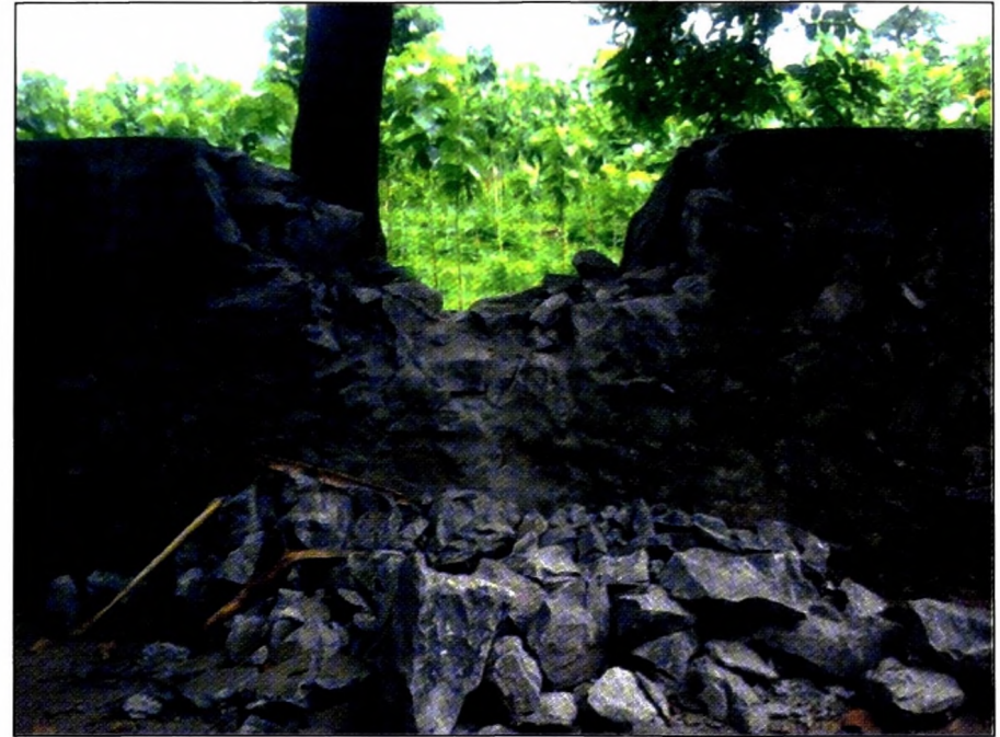
Figure 2. Stone fence damaged by an elephant.
