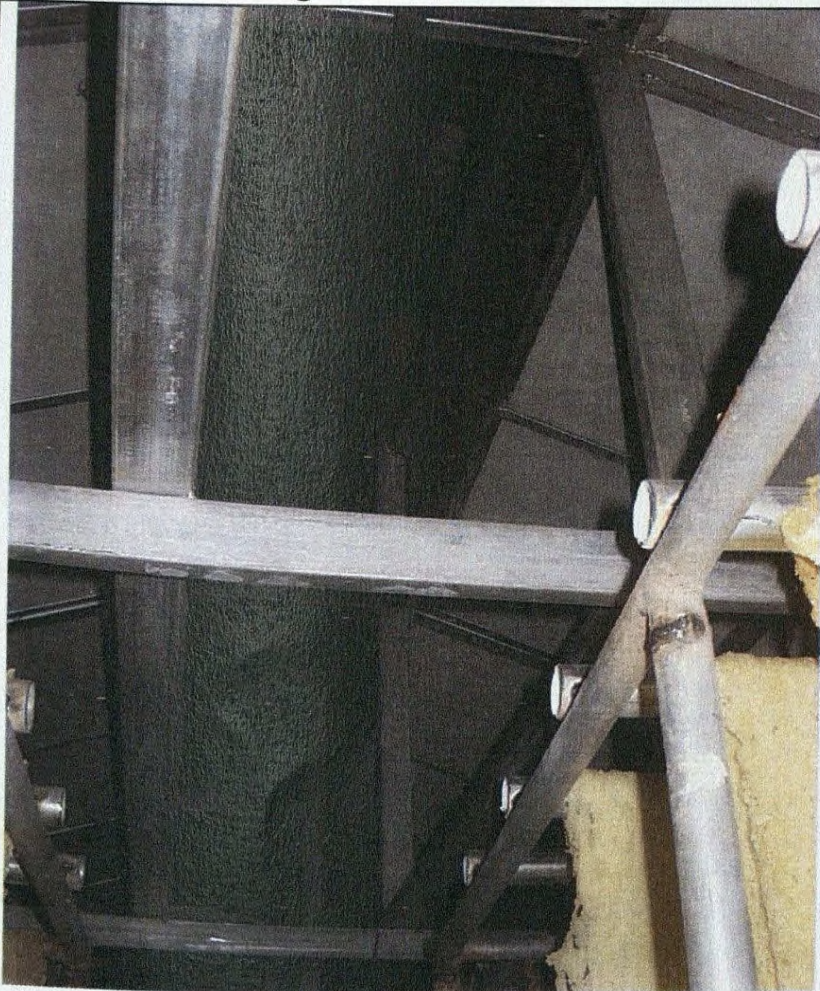
Figure 3: Adjustable ventilator system in inside the hot air drying unit
