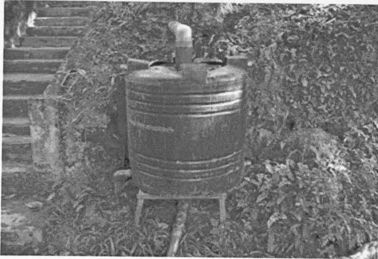
Figure 34: The completed water filtering unit installed behind the Cafeteria
