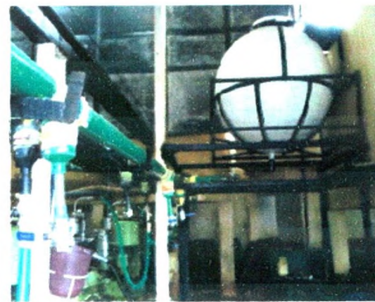
Spherical bulking Tank
