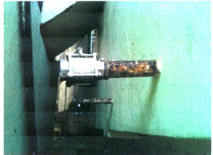
Outlet valve above the bottom of tank
