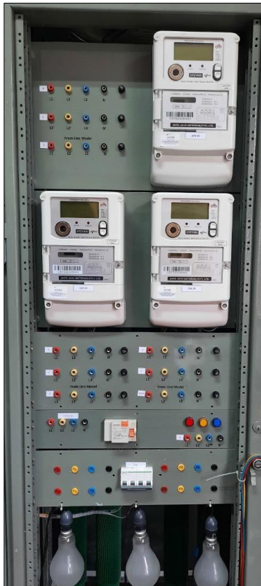
Front panel of the distribution line model designed to test voltage violations and mitigation methods
